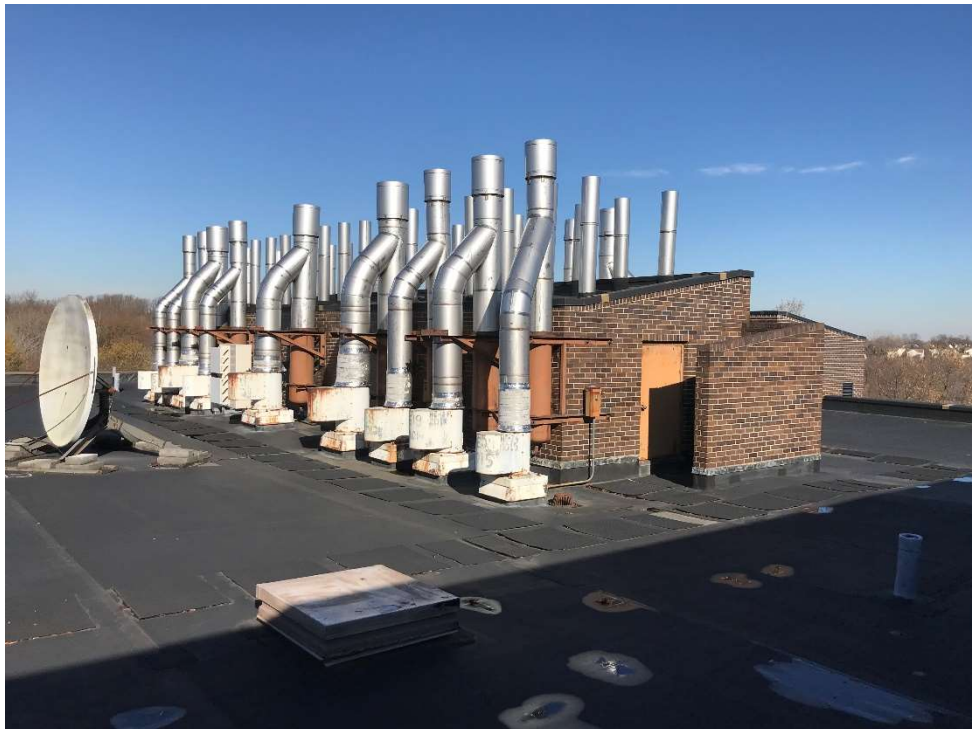
Photo 8 - Laboratory fume hood exhaust ducts and fan units located outside of the Penthouse on the roof level at the Natural Science Building.
