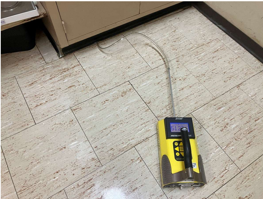
Photo 12 –Elevated mercury vapor readings detected beneath some laboratory casework. Readings collected by inserting the instrument tube in between the opened seams of the covabase and collecting readings from beneath the laboratory casework.
