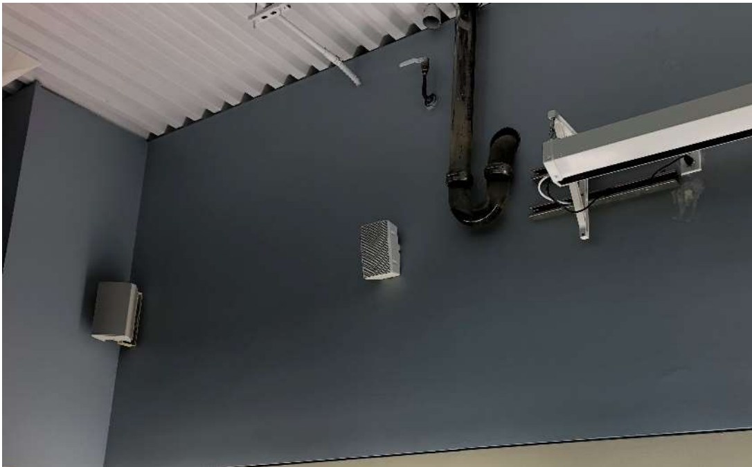
Photo 2 - Laboratory acid waste plumbing line trap with solid contents located within the Natural Science Building.
