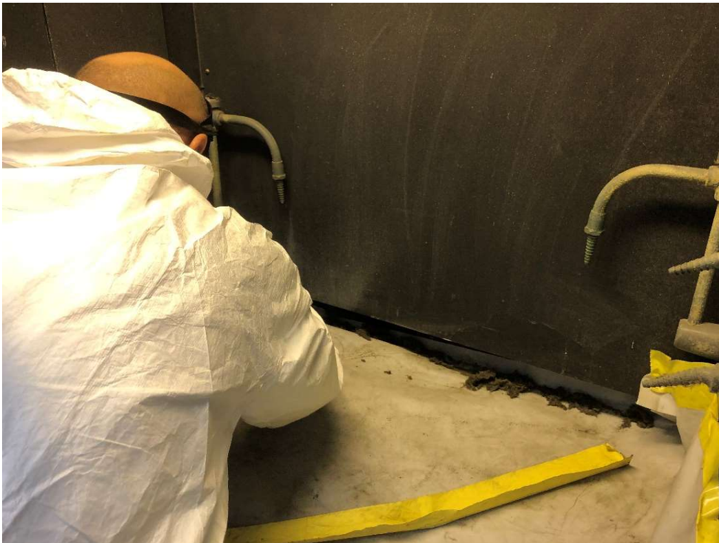
Photo 9 – Collection of dust/debris from within the duct of one of the fume hoods in the Organic Chemistry Laboratory.
