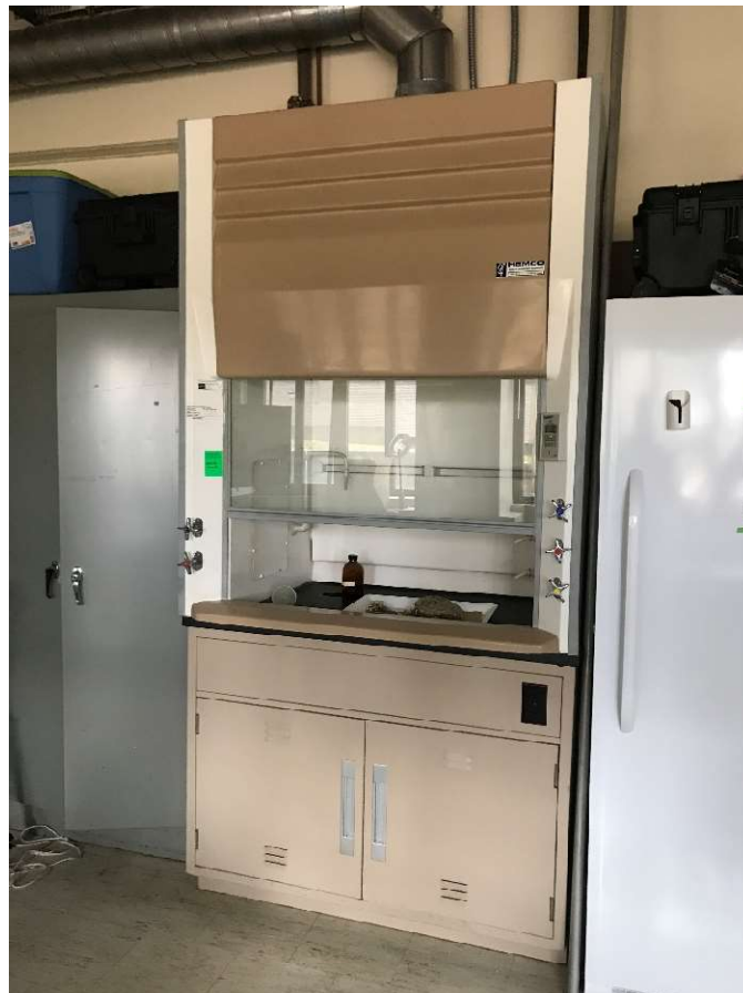
Photo 4 – One of the newer laboratory fume hood exhaust units (circa 1995) within the Natural Science Building.
