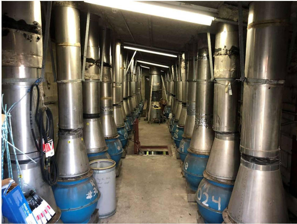
Photo 7 - Laboratory fume hood exhaust ducts and fan units within the Penthouse at the Natural Science Building.
