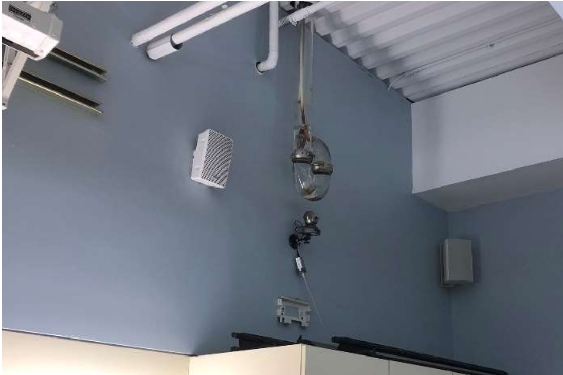
Photo 1 - Laboratory acid waste plumbing line trap with solid contents located within the Natural Science Building.
