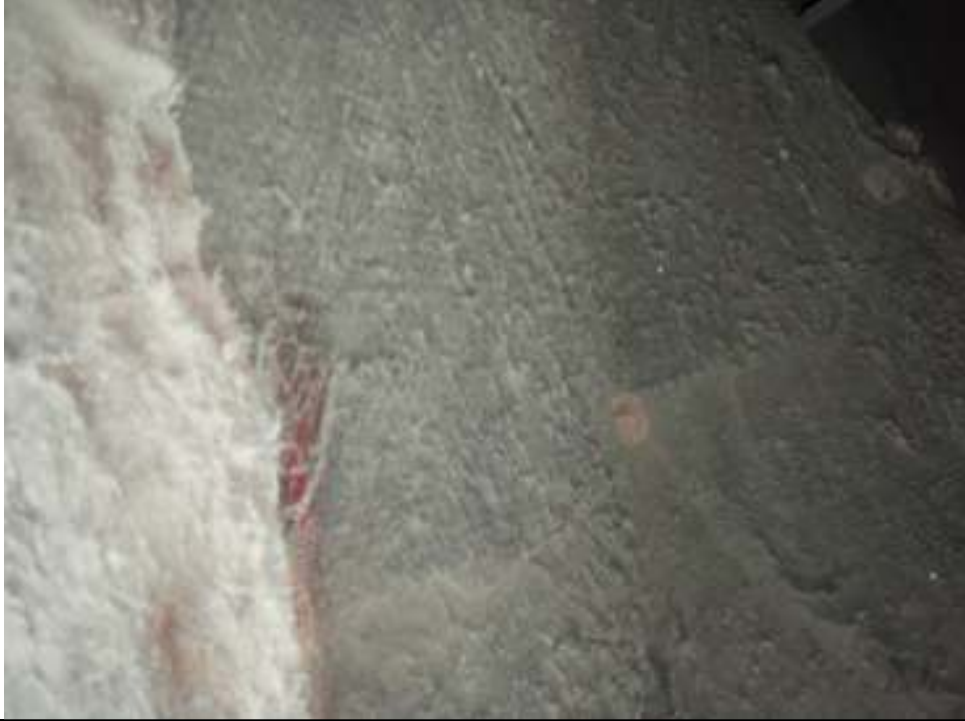
Photo #3 – Typical HVAC unit insulation and mastic (red)
