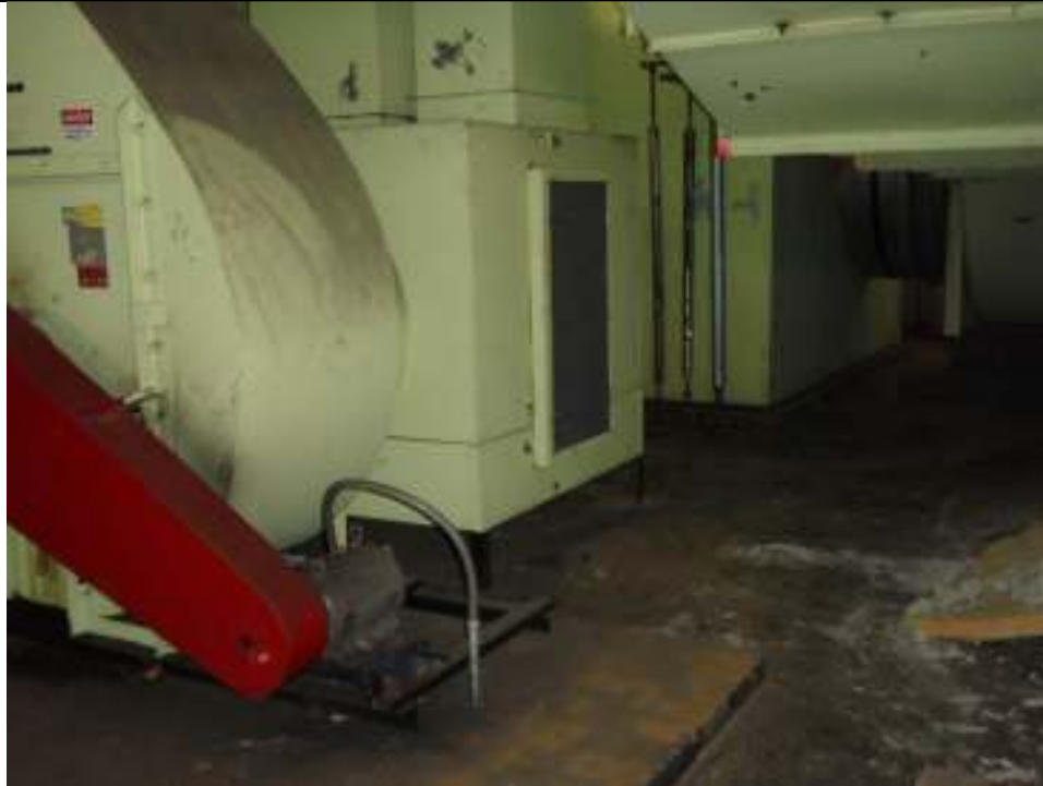
Photo #1 – Typical HVAC unit
