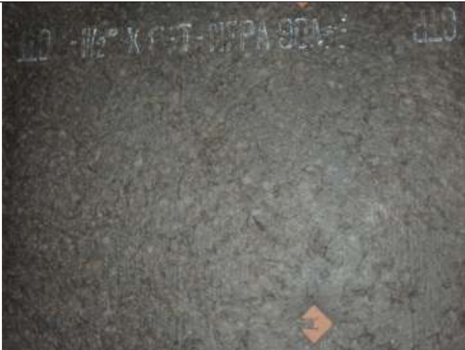
Photo #2 – Typical HVAC unit insulation
